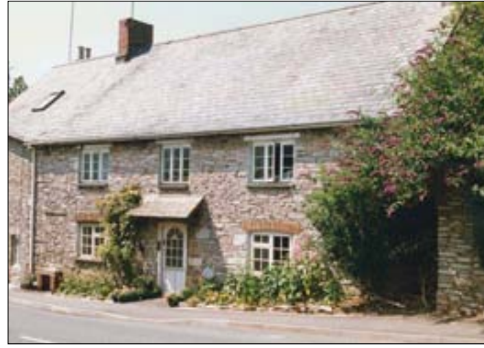
The dominant roofing material in the Area is natural slate. On the majority of historic buildings this is light grey-blue in colour, blending particularly well with the limestone walls
