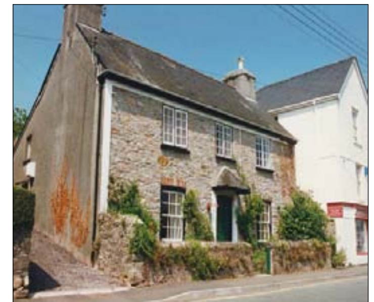
Although 'politely' re-fronted in the 19 th century, the casement windows on the first floor of this dwelling (above) preserve something of its former cottage-like appearance. The painted strips along the eaves and at the corner suggest the stonework front, as well as the side, was rendered over as part of the refronting.
