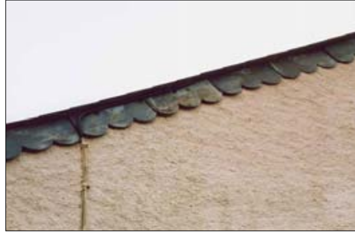
While common on roofs, slate is rarely used to clad walls although its use to protect the verges of gable ends is most attractive and was probably a more prevalent characteristic than it has become today. In this noteworthy example at Paradise House the slates have been scalloped
