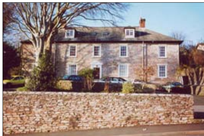
Towards the end of the 19 th century, elevations of exposed stonework were probably fewer in number than today. The Manor is amongst a number of houses that appear to have had their render removed leaving only 'tell-tale' remnants around windows or along the eaves.
