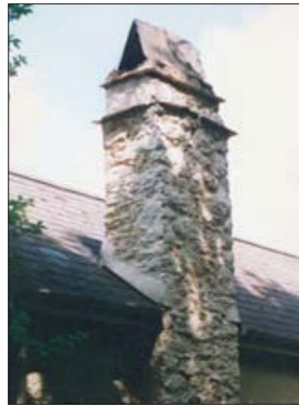
This chimney stack at Turvey is perhaps the most characterful and traditional-looking one in Tuckenhay. The slate 'tent' on the top is especially attractive, and while not listed, the building contributes towards the Area's special interest and character.
