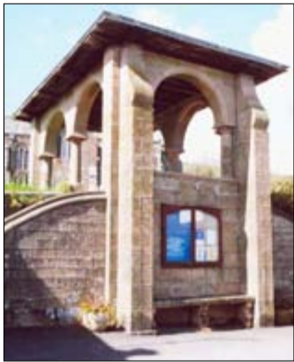
The scale and proportions of the Lychgate are quite remarkable in such a village location and serve to emphasise the significant change in level between the churchyard and the highway that skirts part of its ancient boundary.
